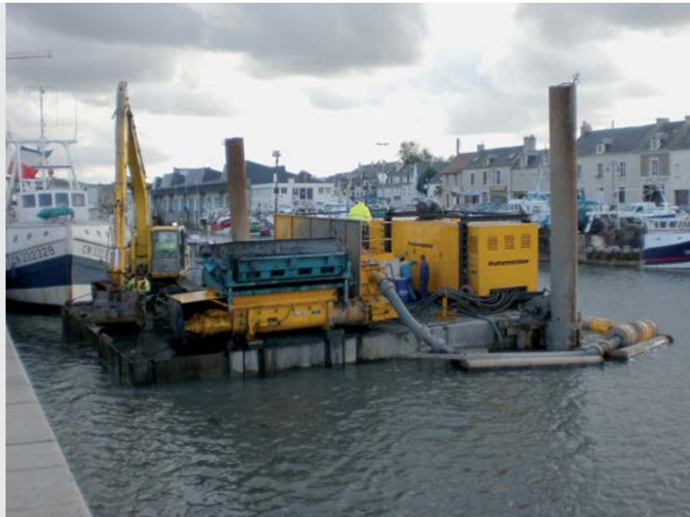
Sludge handling system operating in a canal in France with an S-tube pump and diesel-driven power pack mounted on a ponton
