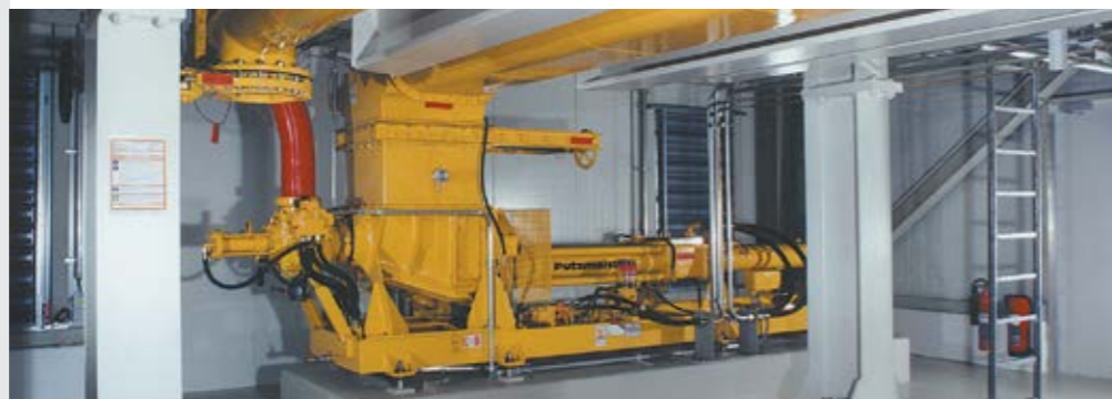
Co-incineration of sewage sludge in the coal-fuelled power plant of Zolling (Germany): KOS 2180
