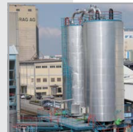
Two 200 m³ storage silos for sewage sludge storage (Pro Rheno, Switzerland)
