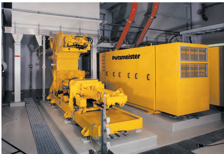
Fig. 42: Receiving bunker with S-tube pump and hydraulic power unit
