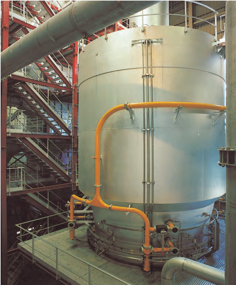
Fig. 31: Sewage sludge distribution with four charging points at the furnace
