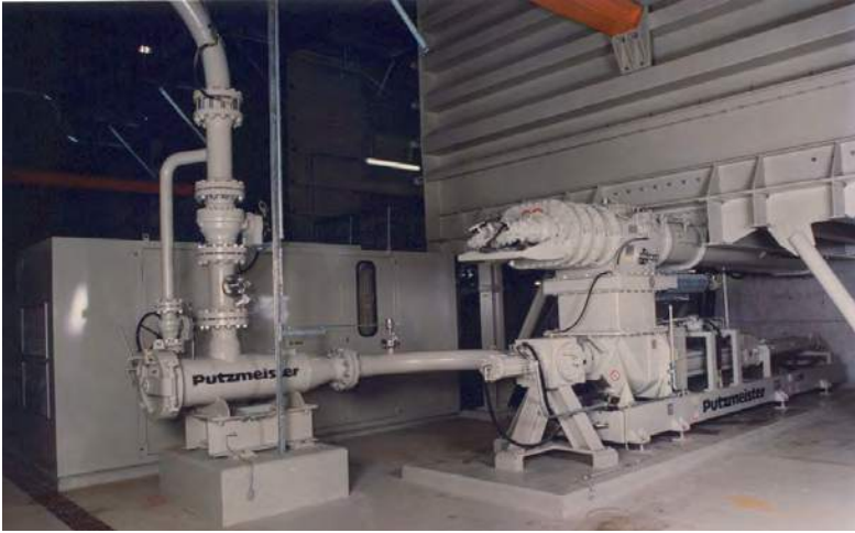
Fig. 39: Screw and piston pump underneath the receiving bunker
