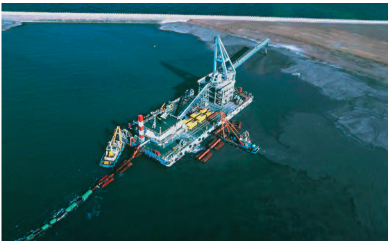
Fig. 147: Sludge supply with barge preparation plant on the vessel stacker conveyor for the prepared medium
