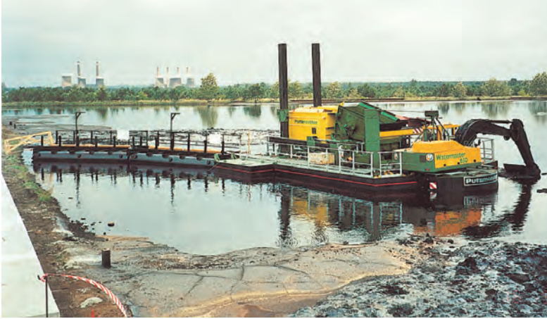
Fig. 59: Remotely controlled operating platform
