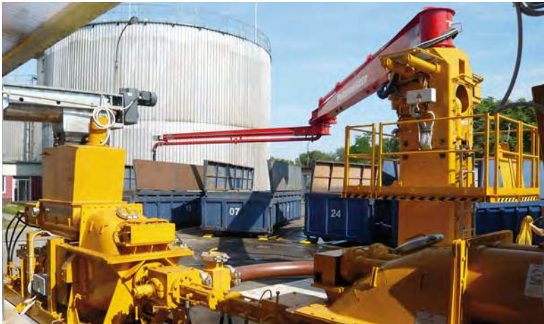
Fig. 82: Waste water treatment plant Prague, Czech Republic
