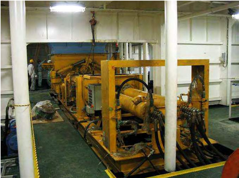
Fig.72: Piston pump- installed below deck
