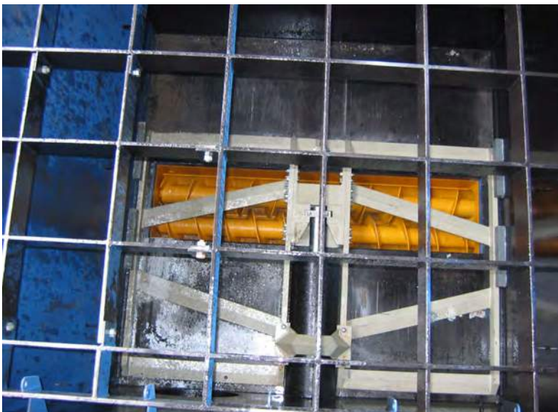
Fig. 112: Look in the bunker with rectangle sliding frame 3.5 x 3.5 m (LxW) and auger feeder (yellow) 2 x 400 mm diameter with 3.5 m length
