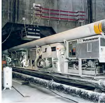
Fig. 64: One of eight muck pumps during the construction of the Euro Tunnel between France and England
