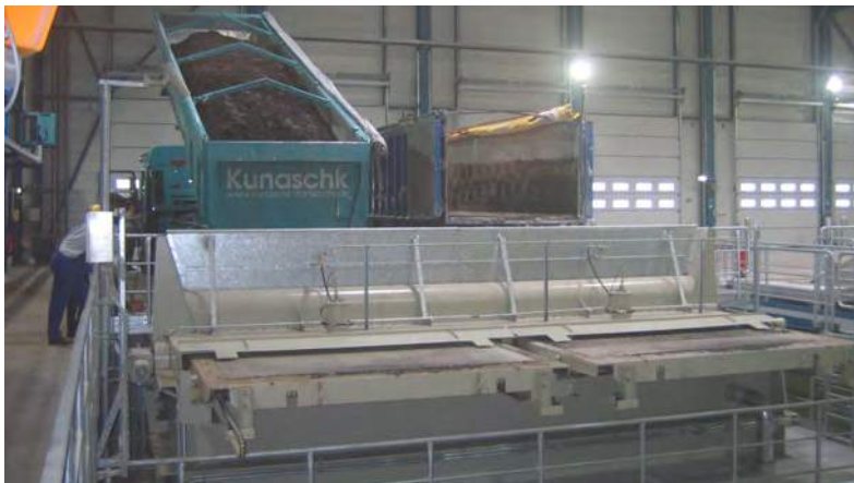
Fig. 38: Receiving bunker for unloading of two trucks
