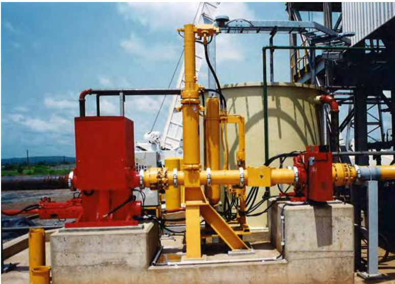
Fig. 128: Automatic pig entry lock for delivery line cleaning (left, red)
