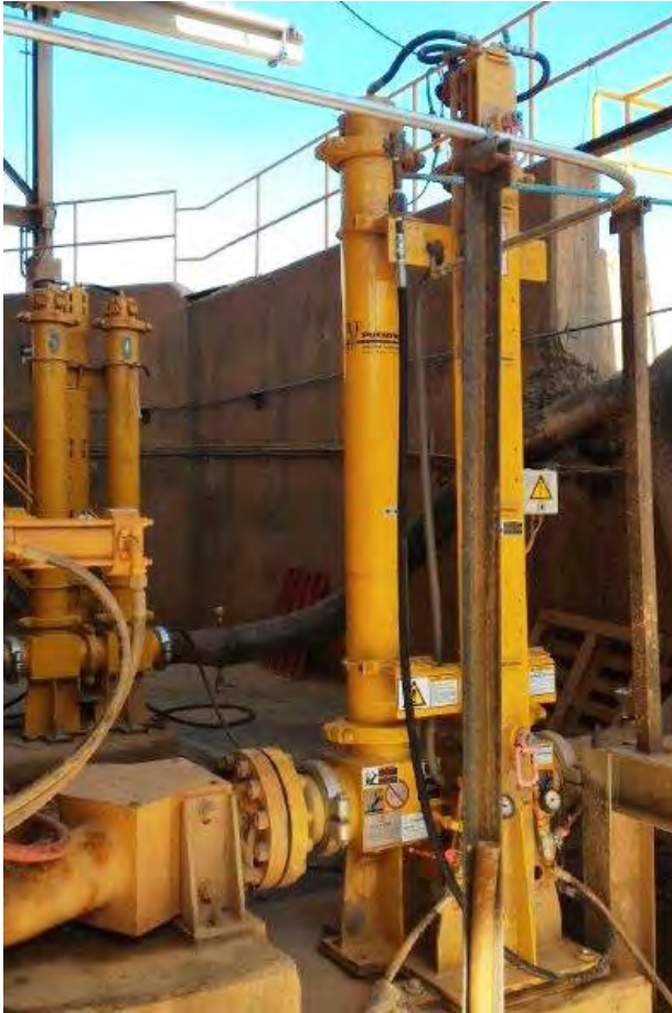
Fig. 140: Installed VPD dampening system for tailings handling
