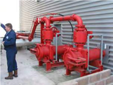
Fig. left 123: Two separators installed directly after the foreign sludge acceptance
