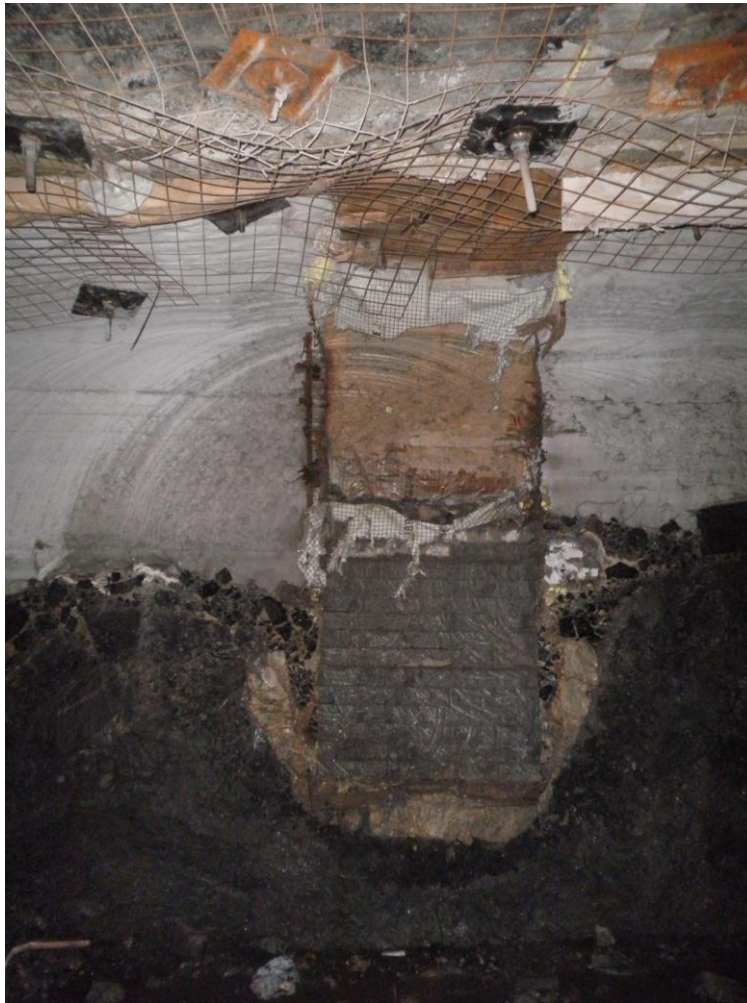
Figure 7: Fibre-cribs mid-shear (after PDRR 20 was backfilled) and two shears were taken into the failed pre-driven recovery road
