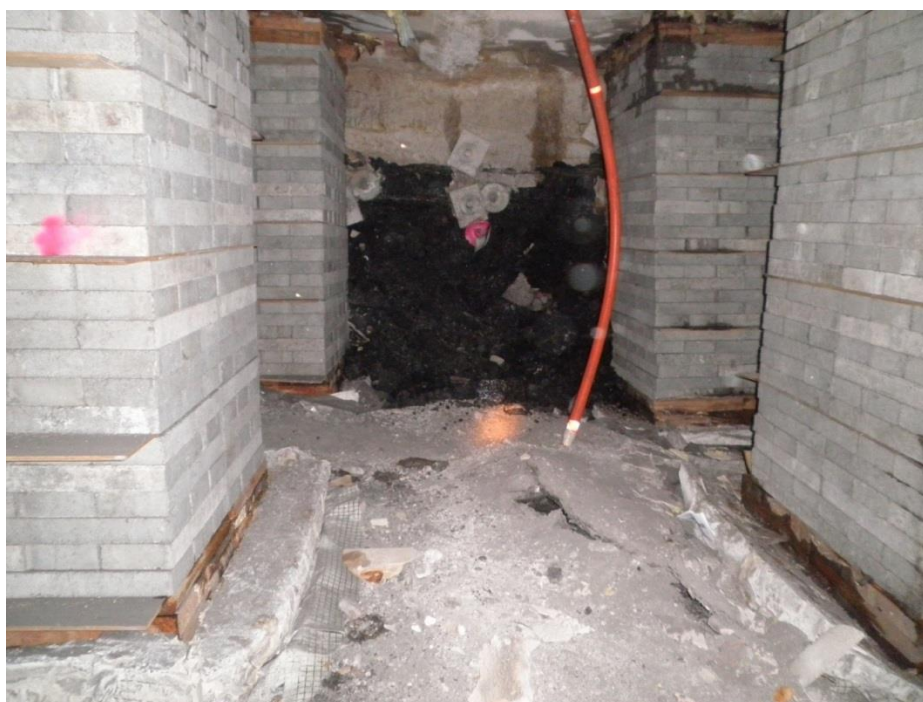
Figure 6: Fibrecrete cribs starting to punch into weak floor
