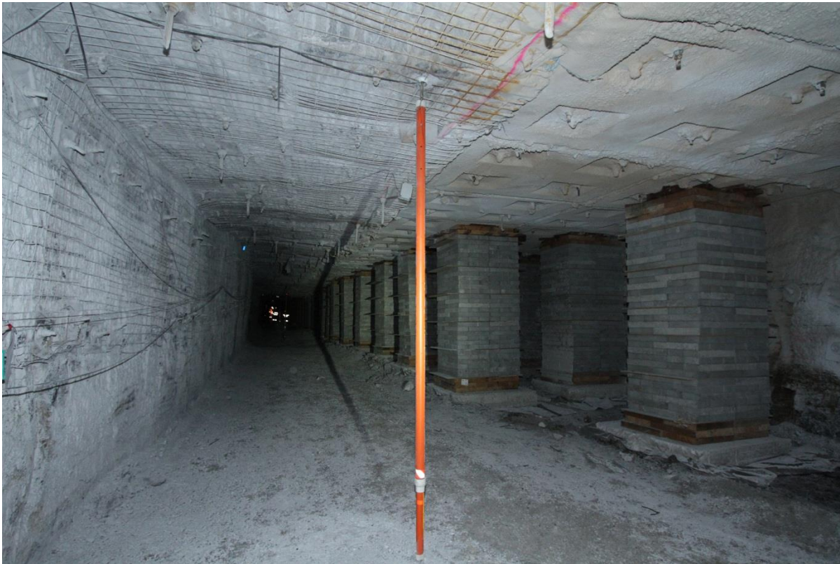
Figure 3: Fibre-cribs in PDRR 20 prior to floor heave event
